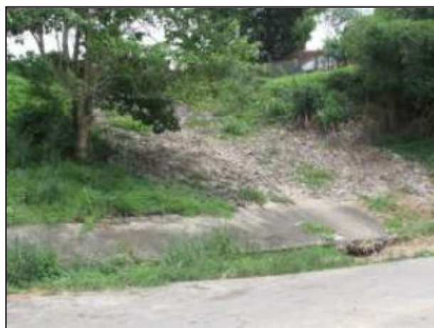
Figure 7c Right wing of the successful slope-stabilization works at the Marina in Calabar. (Photo credit: Ukorebi, U. A.)
