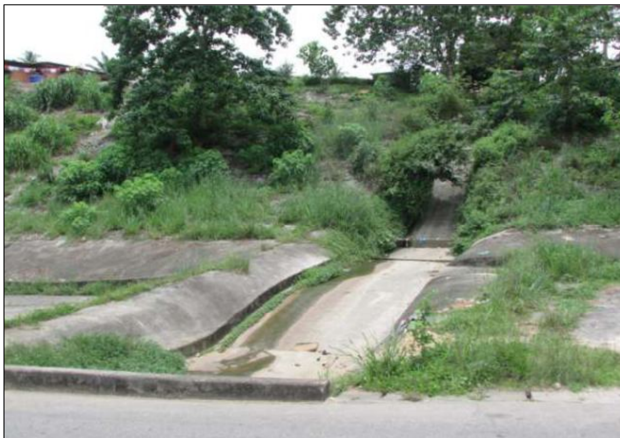
Figure 7a: Example of successful slope-stabilization works (executed by stone-pitching) at the Marina in Calabar. (Photo credit: Ukorebi, U. A.)
