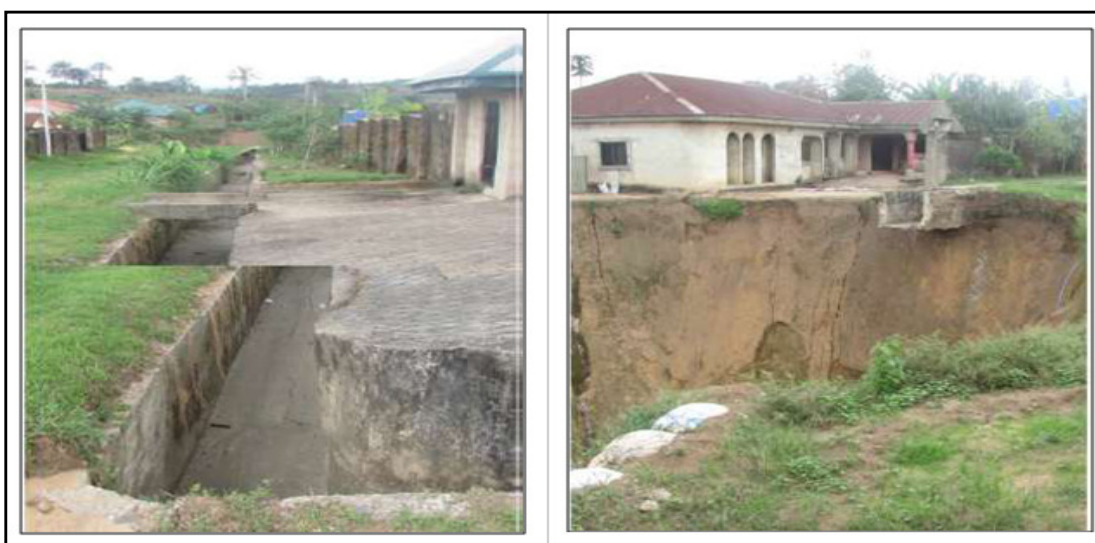
Figure 5b: The huge concrete drain channel that was constructed to convey stormwaters from Sector-B of the study area towards the valley
