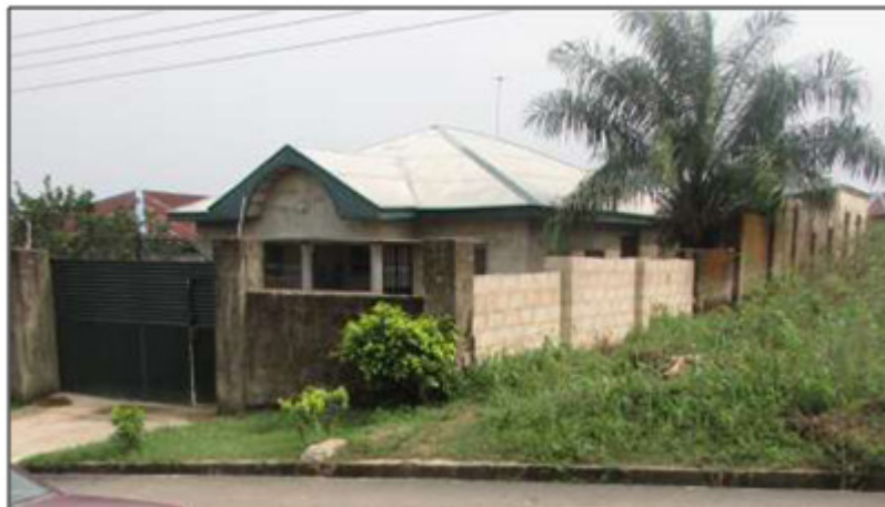
Figure 3b: A part of the fence of another compound, located in the same housing row, was pulled down during the rainy season of 2014. The fresh masonry work on the fence shows the part that was repaired after the incident.
