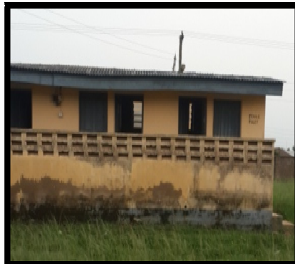
Figure 12: Public Toilet at Federal Polytechnic Ilaro Completed in Less Than 10 Years, Badly Affected by Weather Source: Authors Field Photograph 2017
