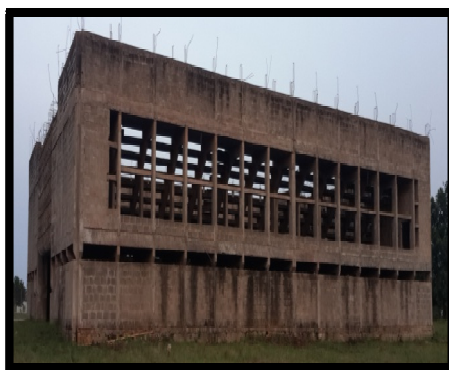
Figure 11: Sport Centre Unplastered Block Wall Abandoned For Over 40 Years at Federal Polytechnic Ilaro. Badly Affected by Weather Source: Authors Field Photograph 2017
