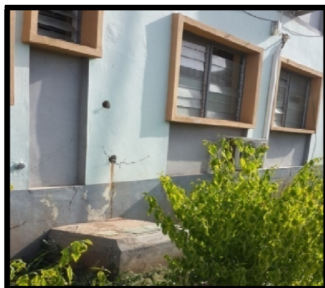
Figure 7: Administrative Building Completed within The Last 10 Years at Federal Polytechnic Ilaro Fairly Affected by Weather Source: Authors Field Photograph 2017
