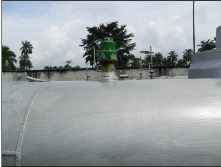
Figure 2: Access valve for insertion of coupon in a 24" pipeline.
