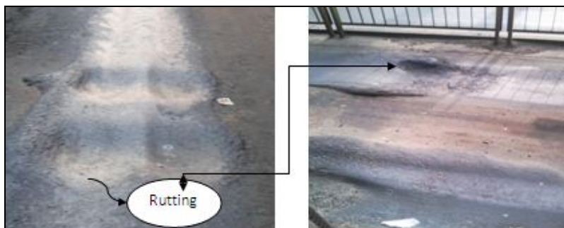
Figure 1: Distresses on the BRTS Bus Shelter; (A) Bhavasar Hostel (B) Valinath Chowk
