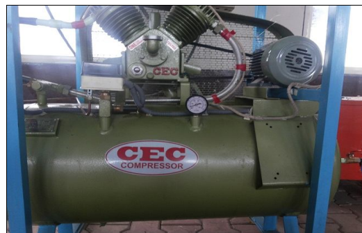
Figure 5: Air compressor unit
