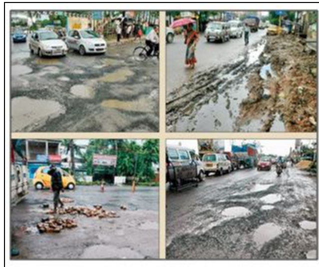
Figure 8: Bad Condition of road surface
