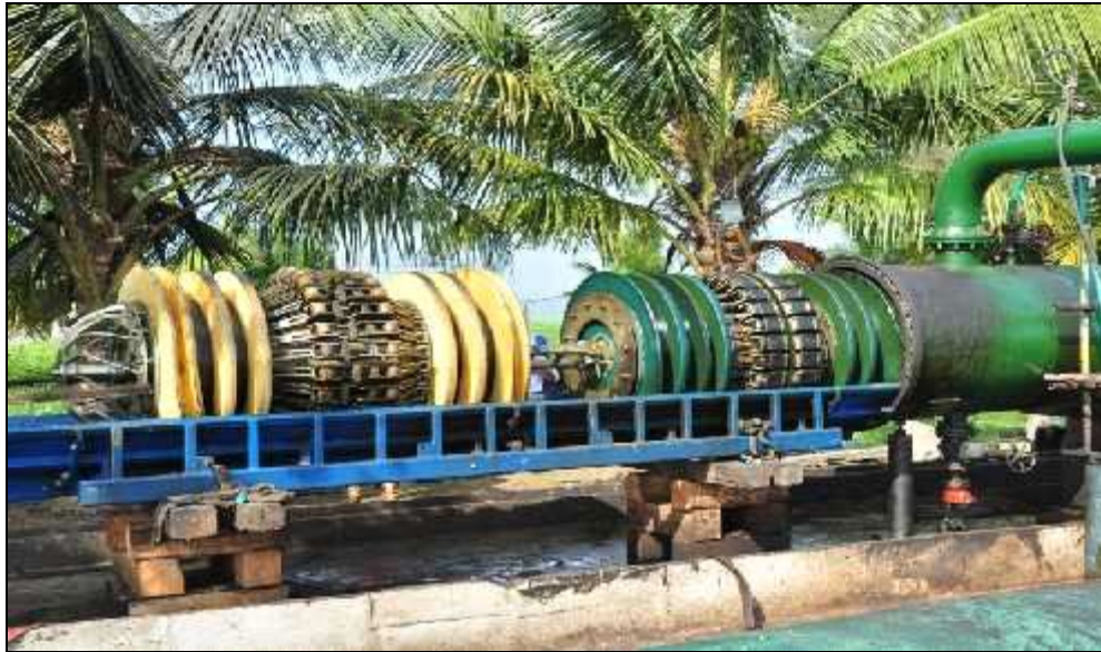
Figure 5: Intelligent Pigging of 48 “ Offshore Crude Pipeline
