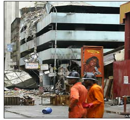
Figure 9: Collapsed office building, possible result of poor Construction standard, Lagos, Nigeria (bbc.co.uk)
