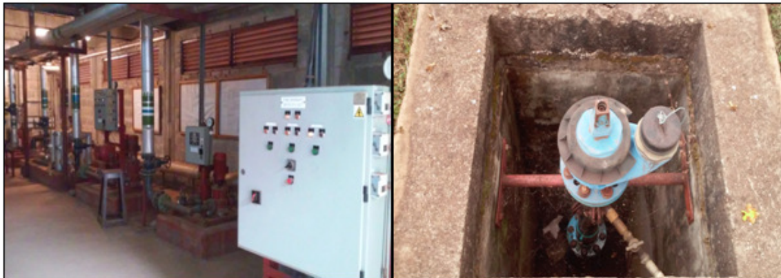
Figure 7: Central control system for hydrants
