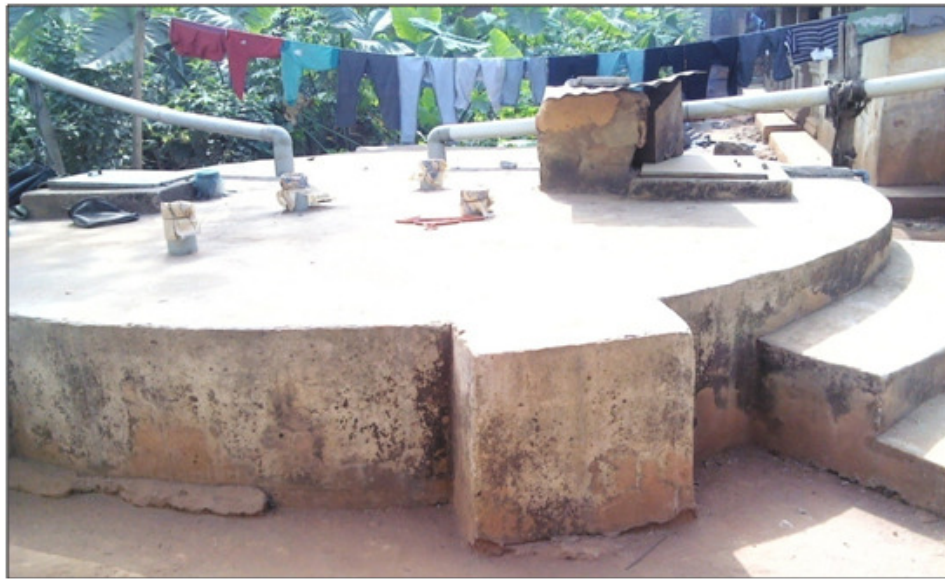
Figure 8: Underground water tank with proper water channeling in one of the households in the study area
