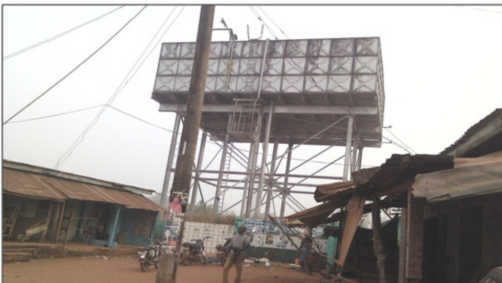
Figure 9: A non-operational water project located at Ekeubahaeze market square Awo Idemili in the study area
