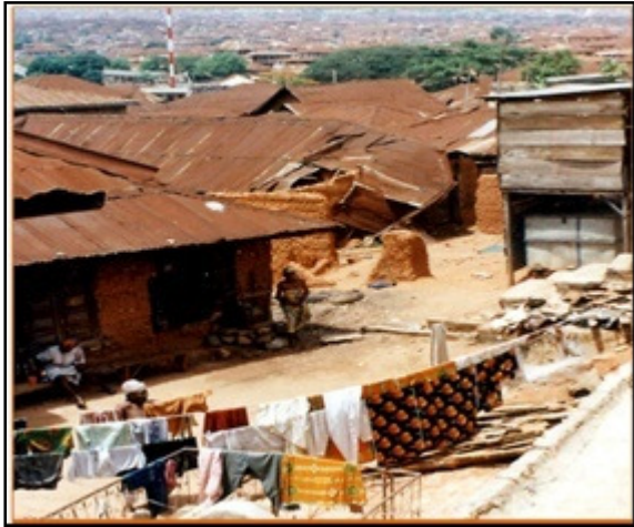
Figure 3: building condition in study area
