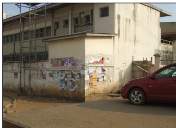
Figure 8: Photographs showing Indiscriminate pasting of posters on offices in Tema Metropolis
