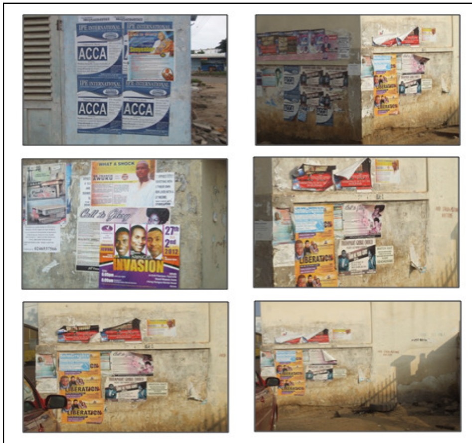
Figure 4: Photographs showing Indiscriminate pasting of posters on buildings in Tema Metropolis
