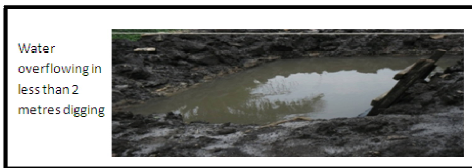
Figure 5: Overflow of a Pit Still Being Dug for Aseptic Tank in Bisseke, Bonaberi Source: Kah Evans
